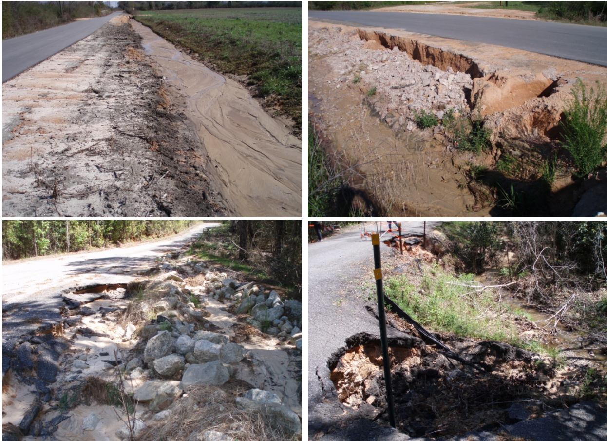
Figure 1. Catastrophic Crossing Failures Following Road Paving in CPB Portions of Holmes and Washington Counties
