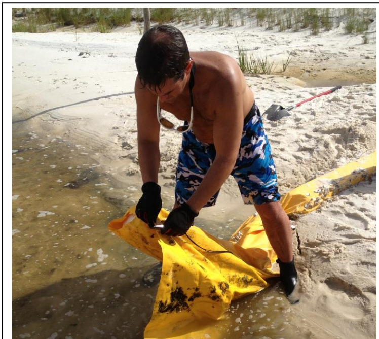
Fig. 58 – Maintaining the barrier requires much maintenance due to being buried by storms
