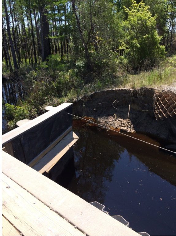
Figure 2. Complete erosion of the bank behind the south wing wall occurred during an extreme event in April 2014.
