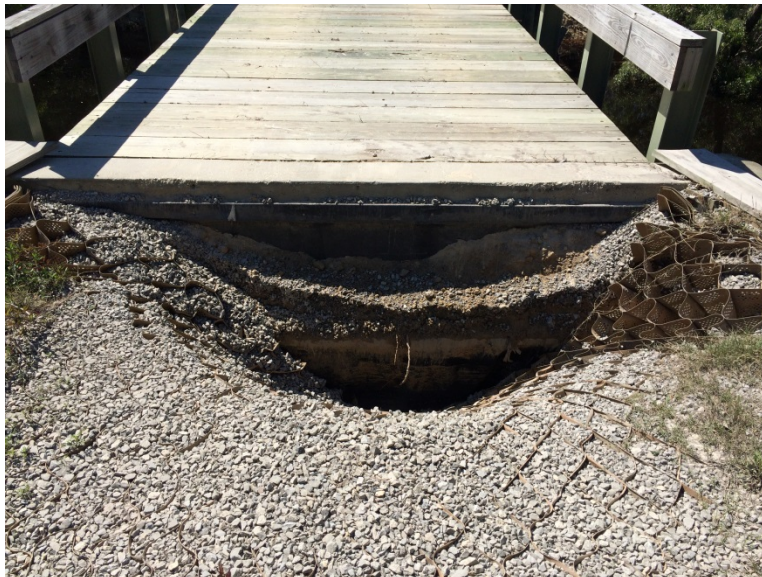
Figure 3. The extreme event of April 2014 caused piping of material on the north wing wall.
