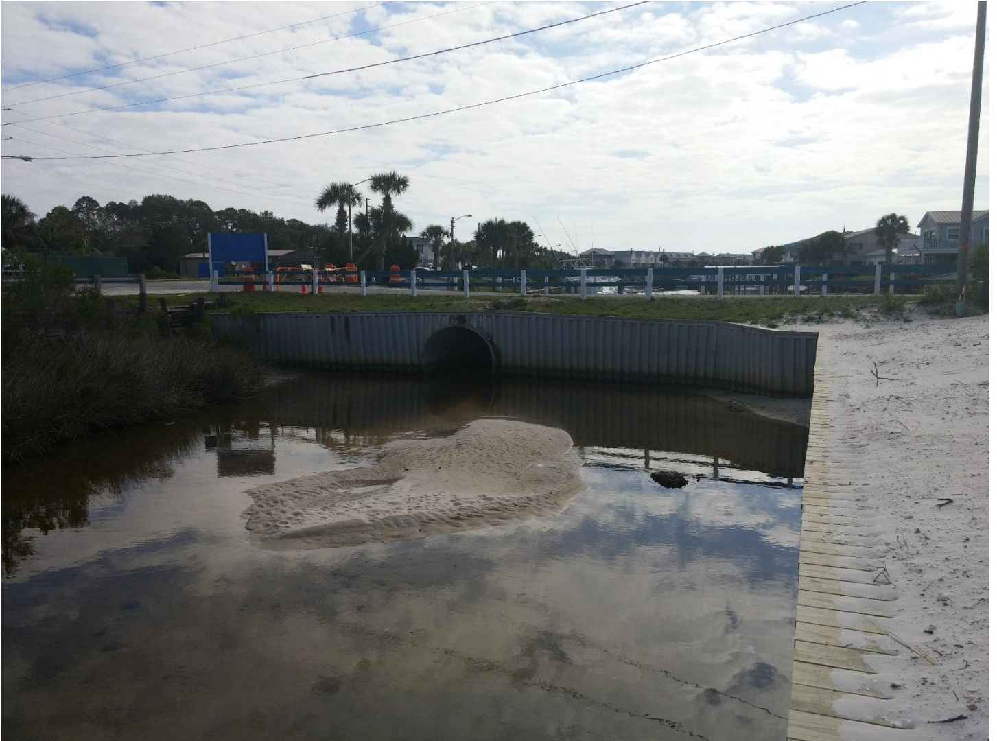
Sedimentation build-up & erosion at the culvert on west-side of Canal Parkway.
