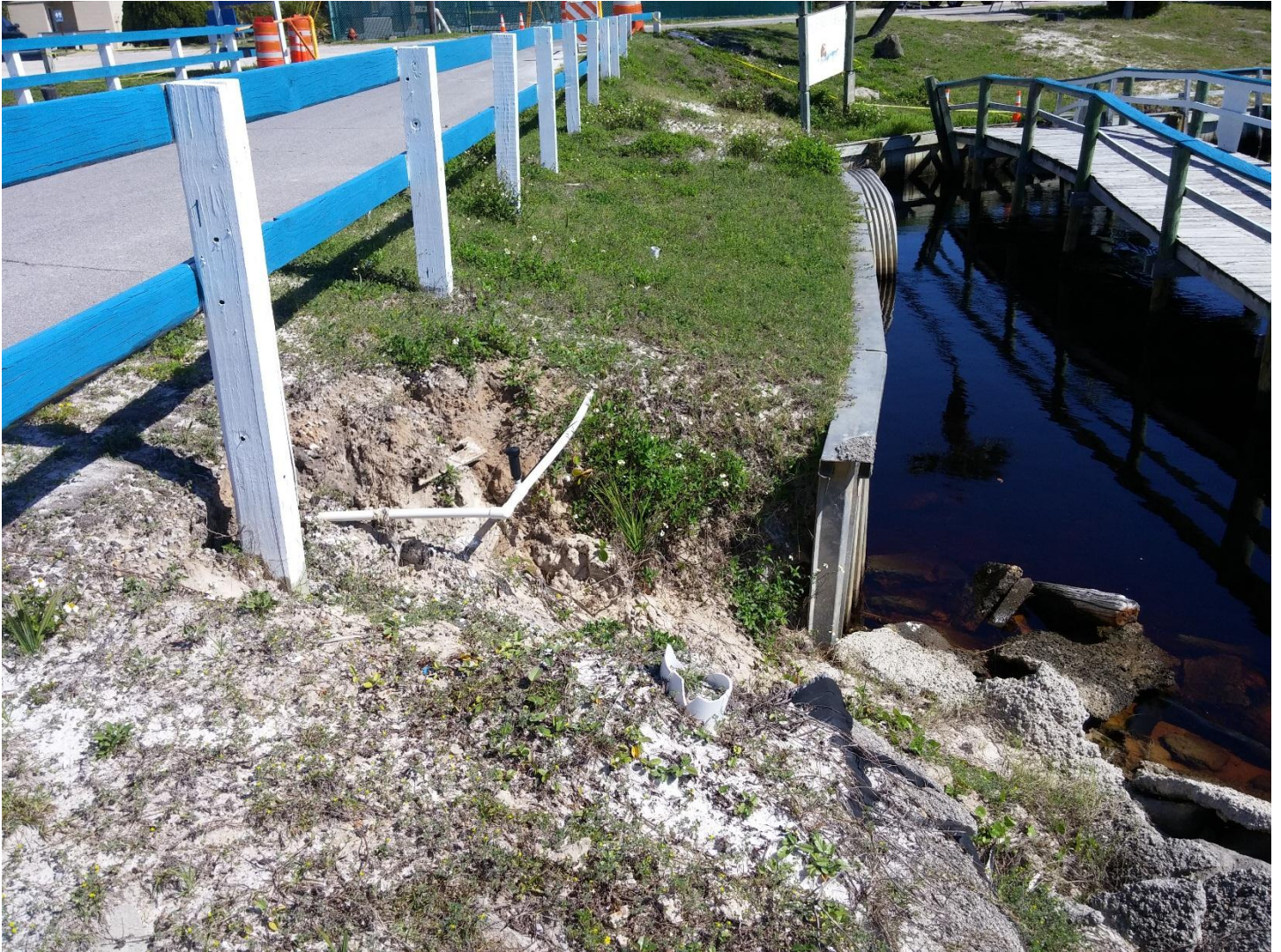
Failing slope & erosion on east side of Canal Parkway.
