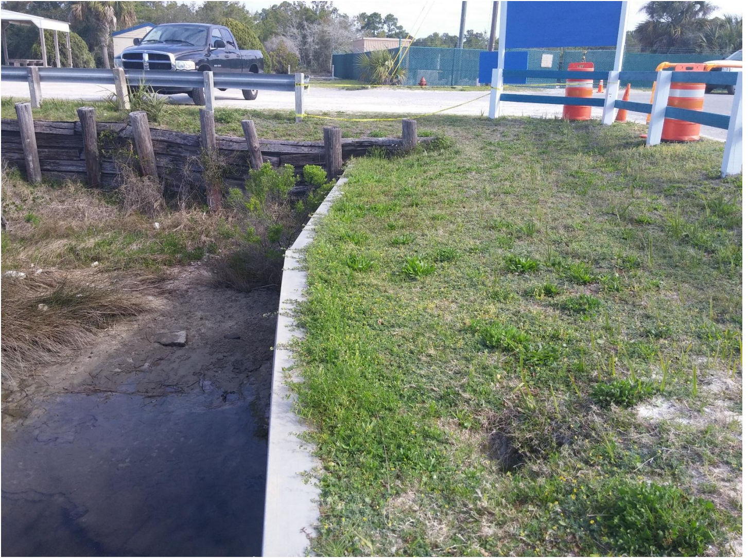
Erosion & dilapidated retaining walls. West side of Canal Parkway.
