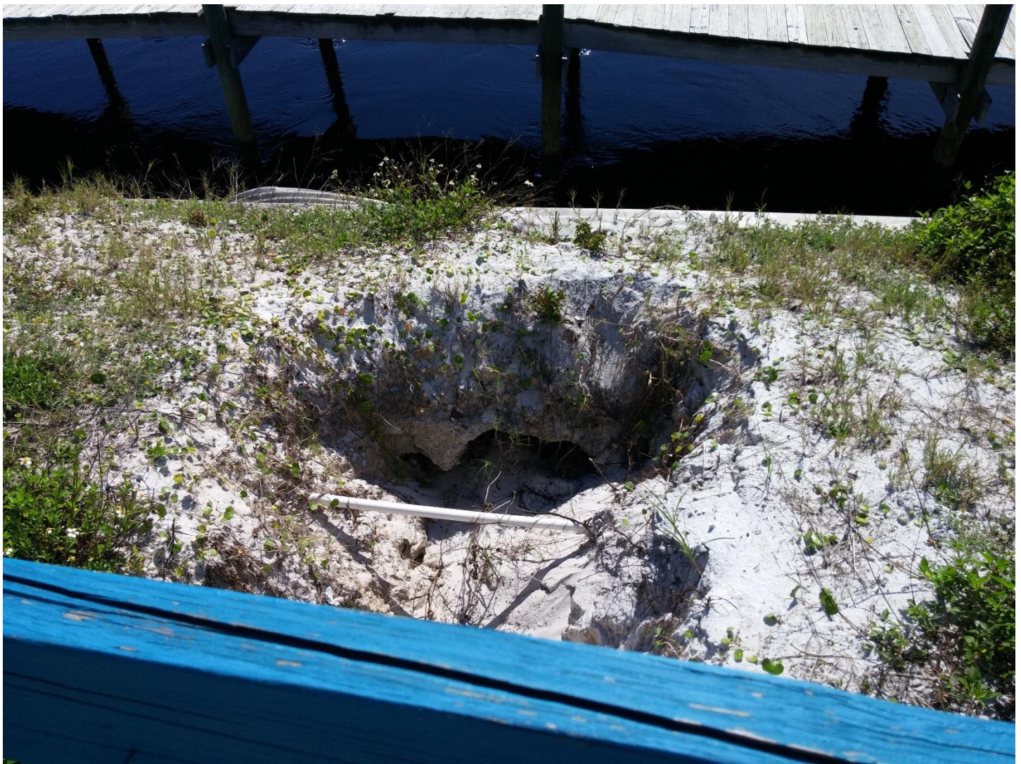
Erosion at culvert on east side of Canal Parkway.
