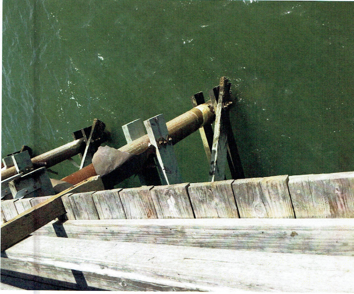
PHOTOGRAPH I – DELAMINATED UV COATING ON FIBERGLASS PILES
