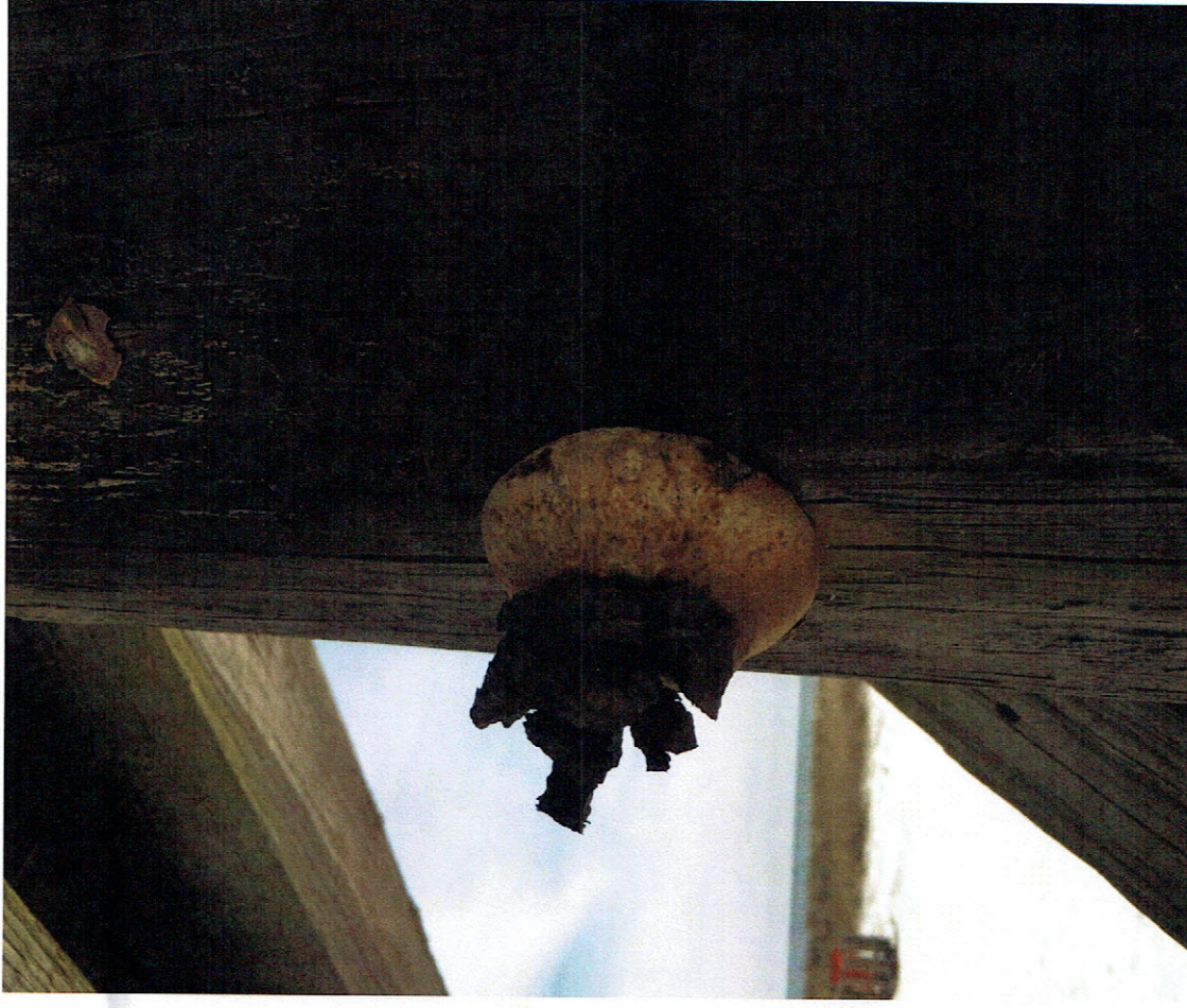
PHOTOGRAPH F – RUSTY HARDWARE
