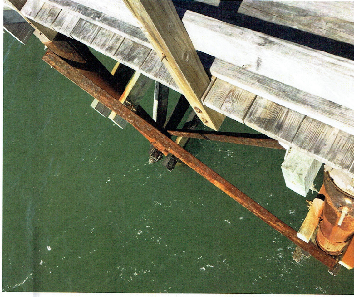
PHOTOGRAPH H – RUSTED BRACING AT "T" SECTION
