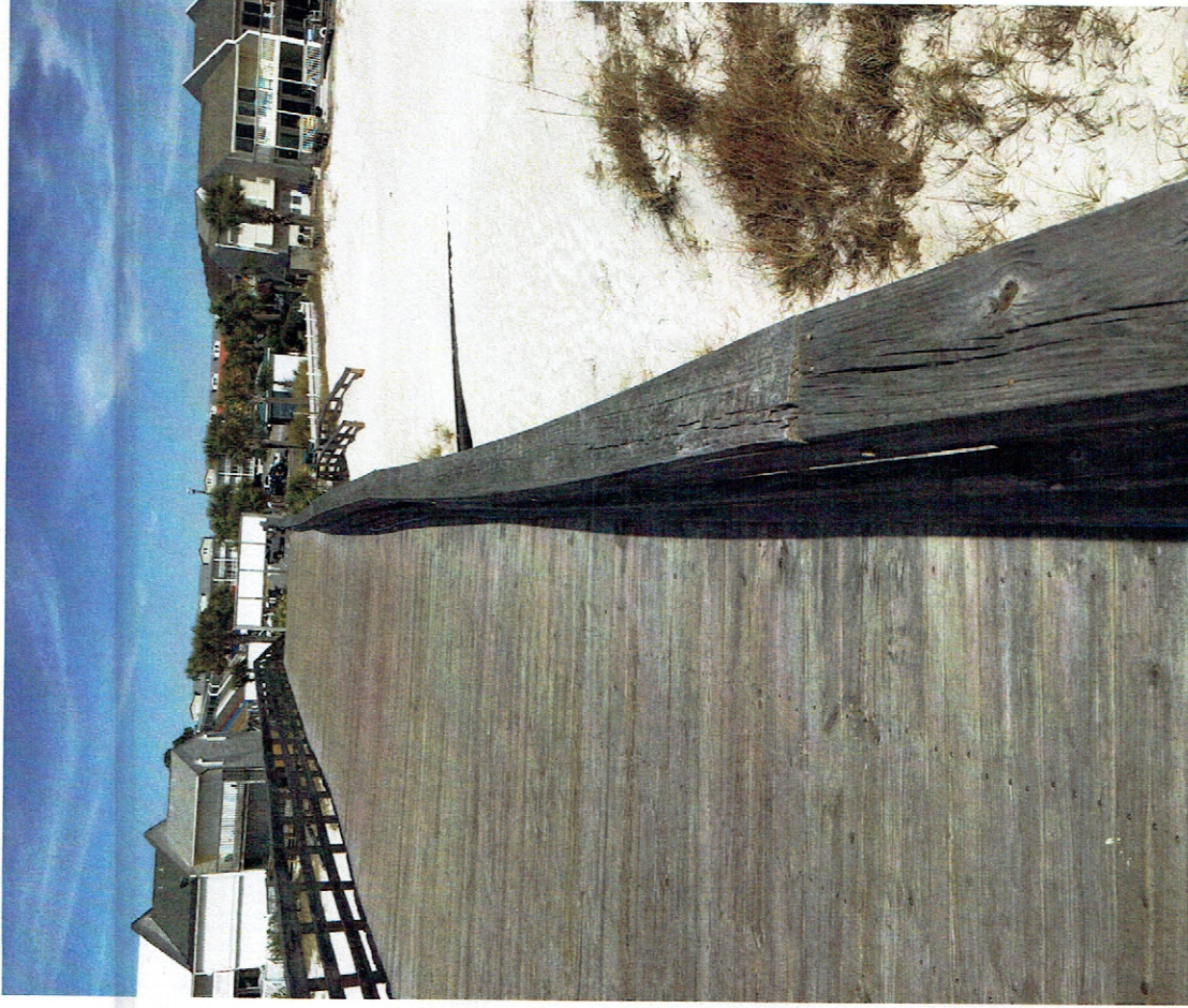
PHOTOGRAPH E – ALIGNMENT & ELEVATION ISSUES
