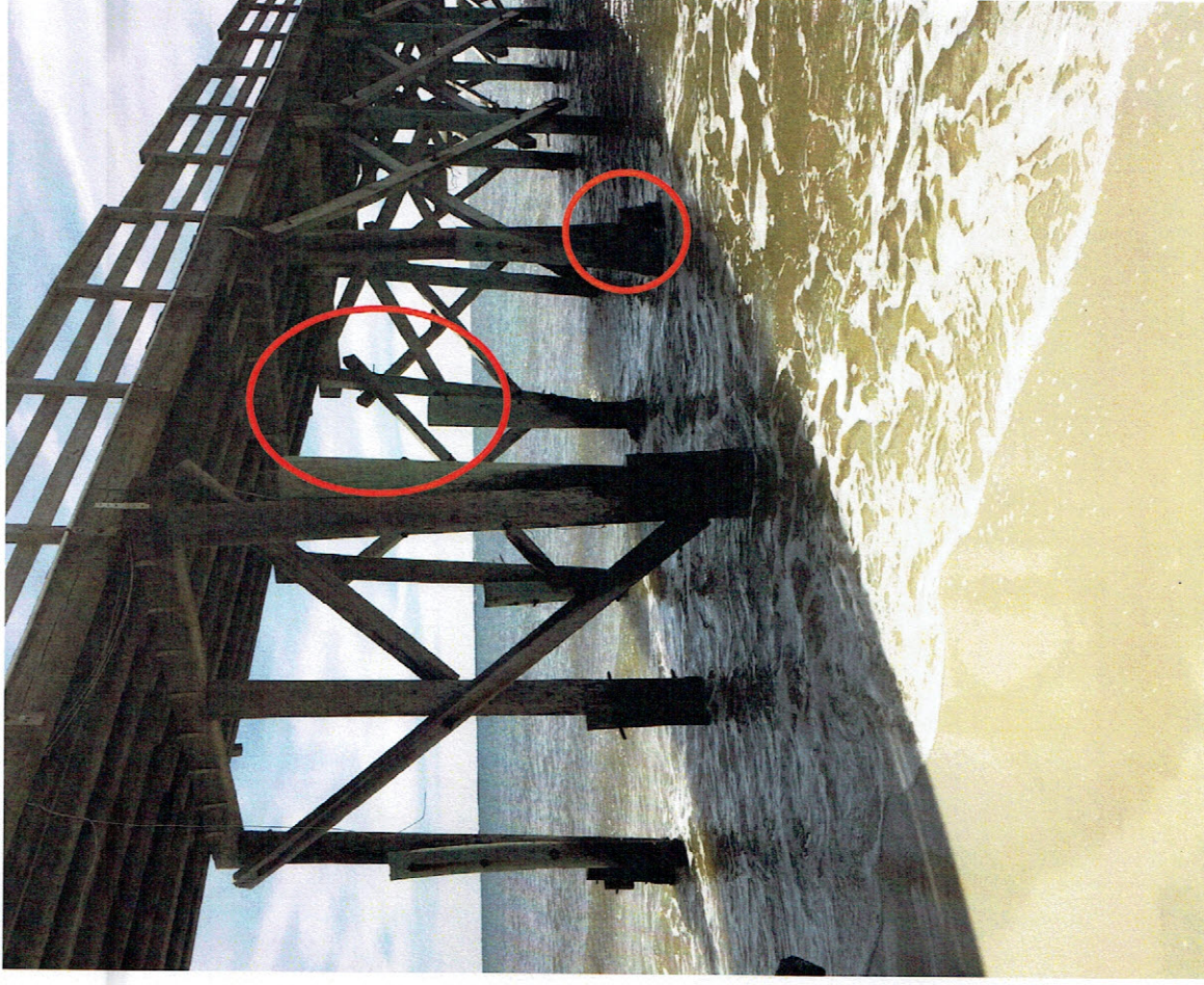
PHOTOGRAPH J – MISSING PILES & SHODDY PILE REPAIRS
