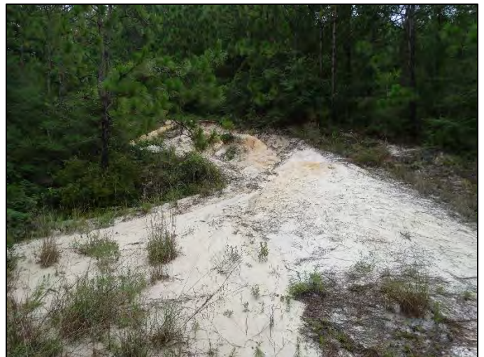
Above: Erosion on the west side of the boardwalk, between the shoreline and the park entrance.
