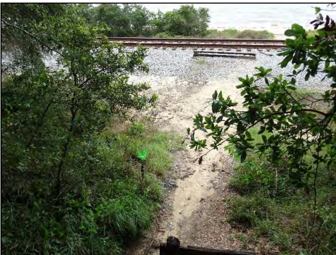
Below: Continuation of the erosion gully shown above.
