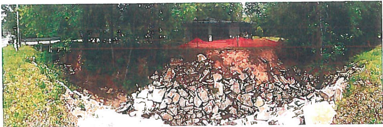
Panoramic of drainage erosion impact to private
