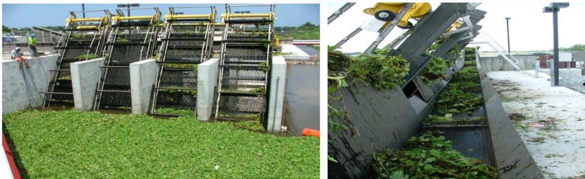
Figure 27. Photographs of the Main Relief Canal Stormwater Treatment Facility. The self cleaning screens capture debris and vegetative material and dump it onto a conveyor that discharges the material into dumpsters. Photos courtesy of Indian River County (Turning the Tide 2008).
