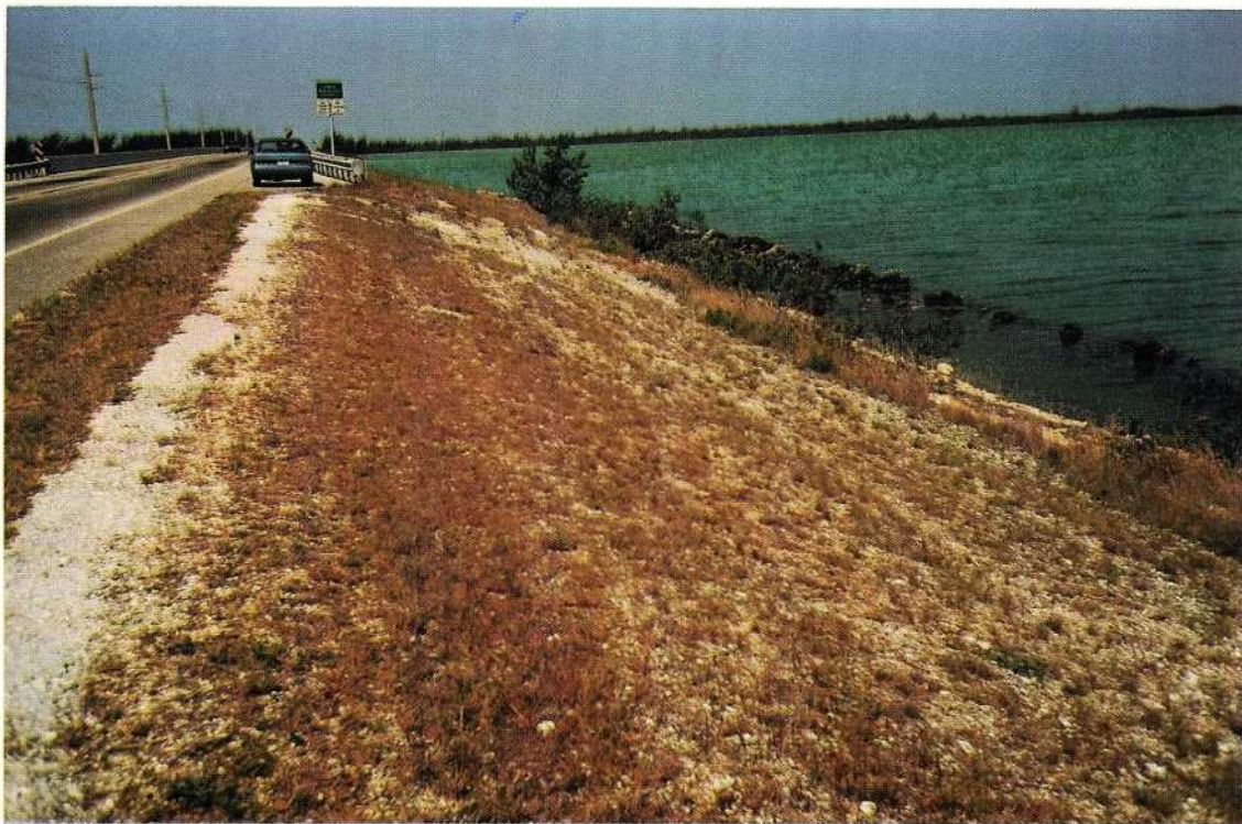
Figure 17. Lower Sugarloaf Channel, erosion limiting revegetation, Miami Gulf side, view west, 5/93.
