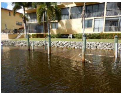
Figure 1.1 King tide flooding docks in the City of Naples Level Rise
