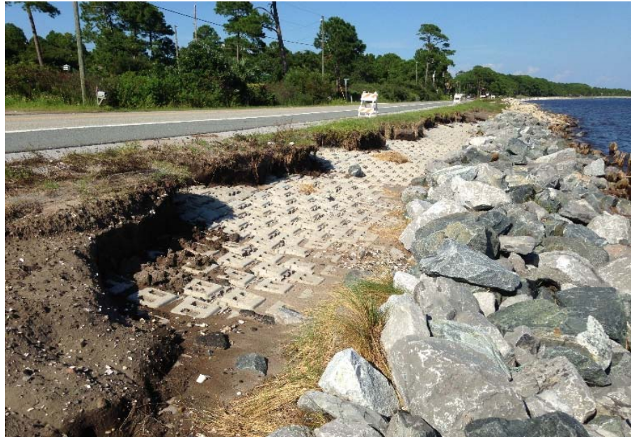
Figure 1: This section of Highway 98 (a designated hurricane evacuation route) requires frequent repairs due to storm damage.
