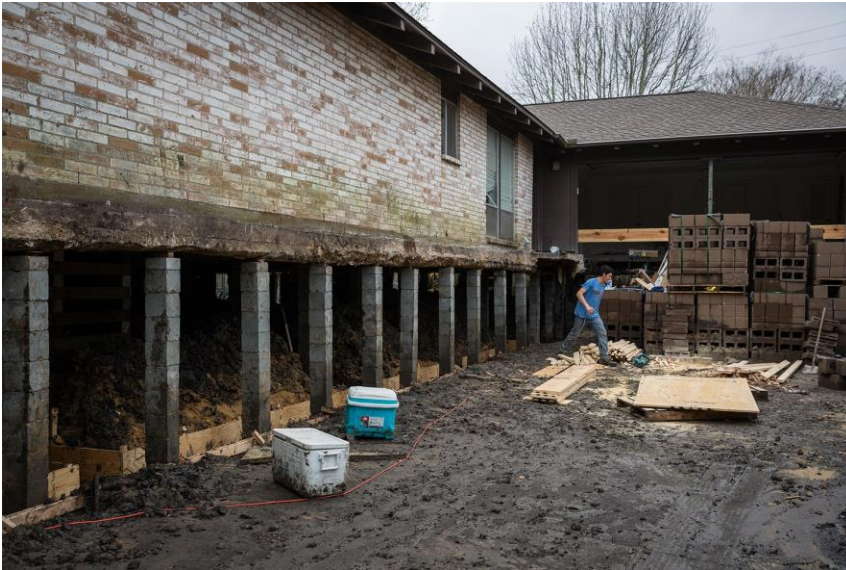
Houston, TX home elevated after Hurricane Harvey
