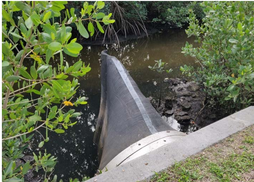
Photograph 4.9 Stormwater Check Valve for Backflow Prevention
