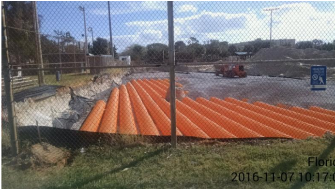
Stormwater system in City Park. (Image courtesy of City of Cape Canaveral.)
