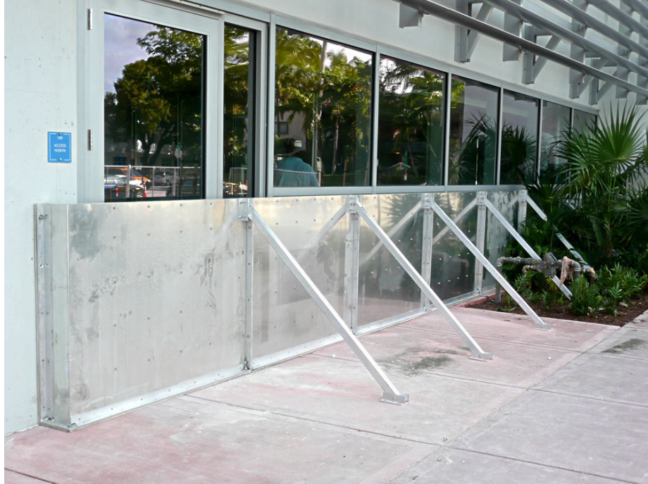
Photograph 4.4 Temporary Flood Barrier Protecting Building Entryway
