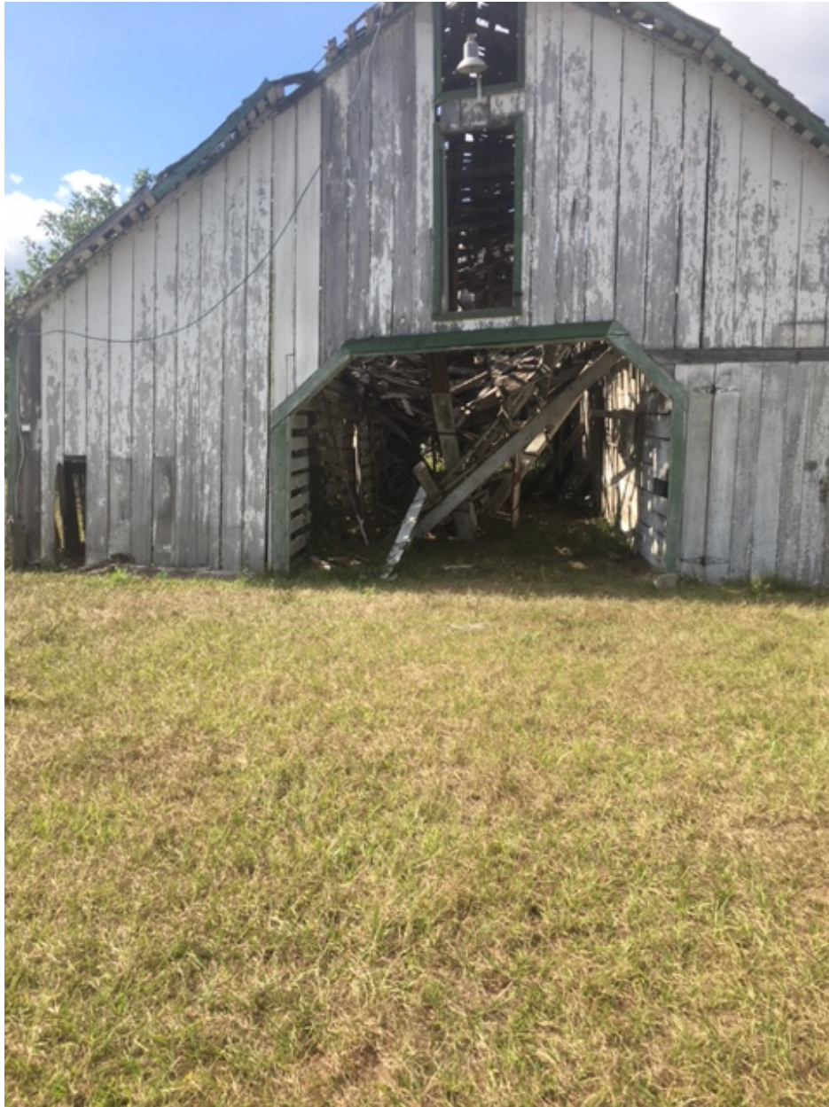
View to the South of the Barn located within Tract No. 19 103-654. Note the deteriorated condition of the structure.
