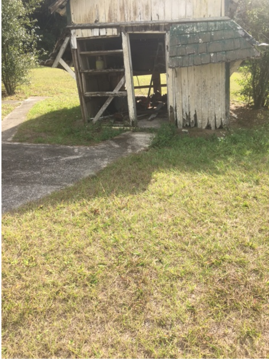
View to the East of Storage Shed located in proximity to the Main House within Tract No. 19 103-654. Note deterioration of structure and miscellaneous solid waste.
