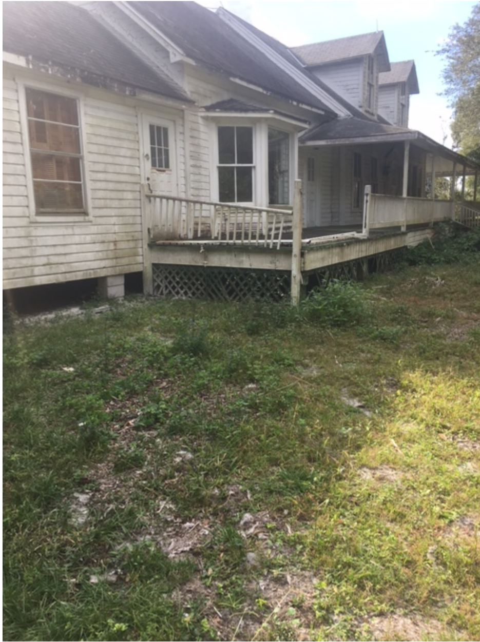
View to the East of Main House located within Tract No. 19 103-654. Note deterioration of the structure.
