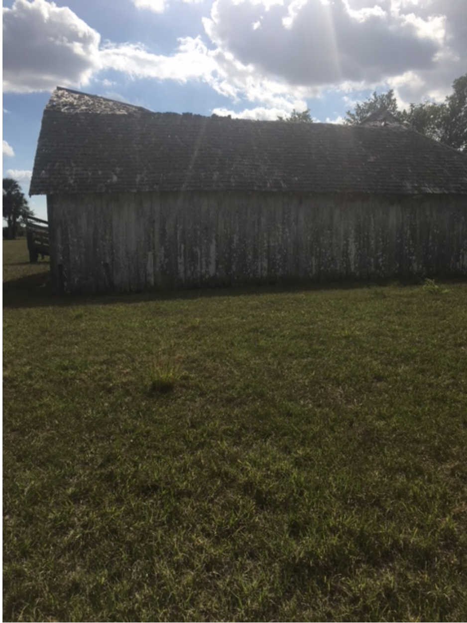
View to the East of the Barn. Note the collapse of the roof.
