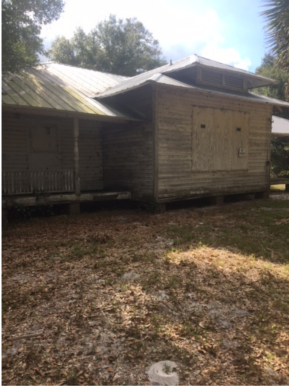
View to the West of School House. Note deterioration of structure.
