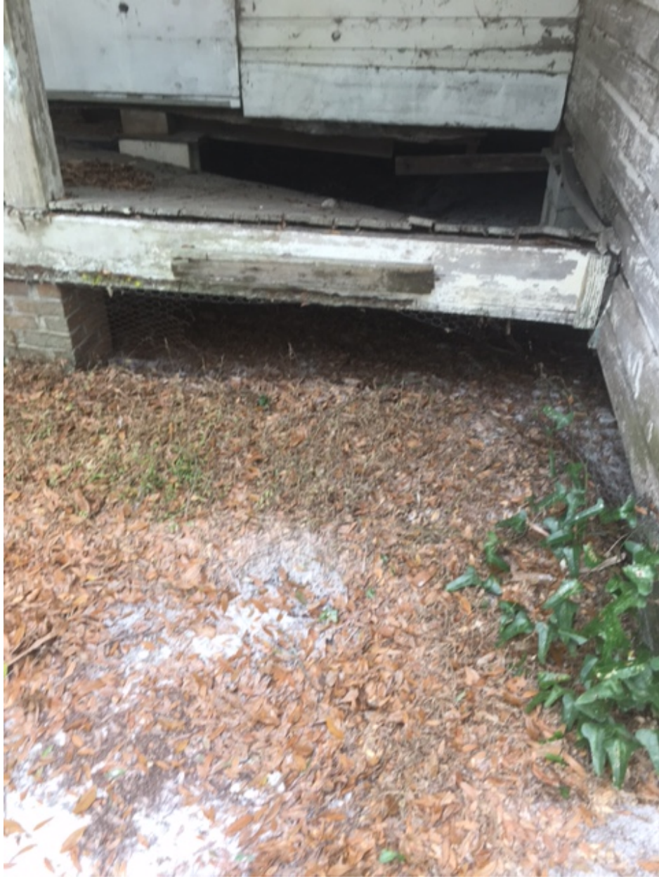
Additional view of exterior of School House. Note deterioration of structure.
