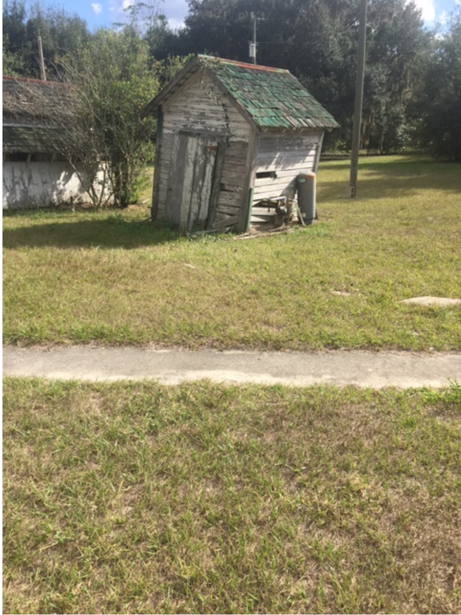
View to the East of Pump House located within Tract No. 19 103-654. Note deterioration of structure.
