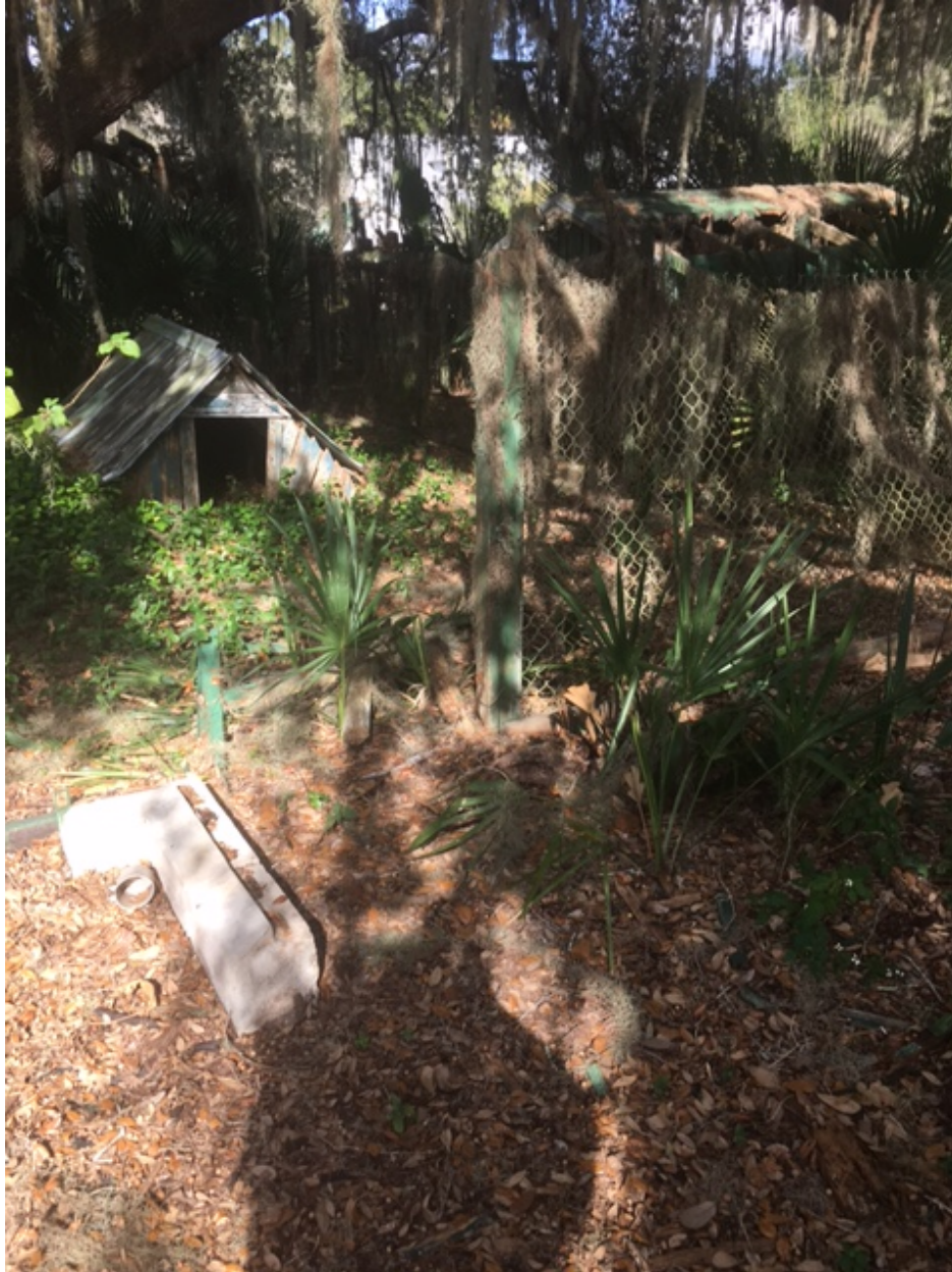
View to the West of the ancillary structures situated adjacent to the Main House (storage sheds, dog pens, etc.) within Tract No. 19 103-654 which have essentially collapsed.
