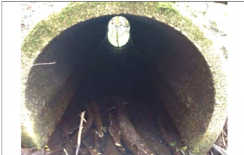
Photo No. 4a. View of debris and sediment in the easternmost culvert (August site visit). View to the north.
