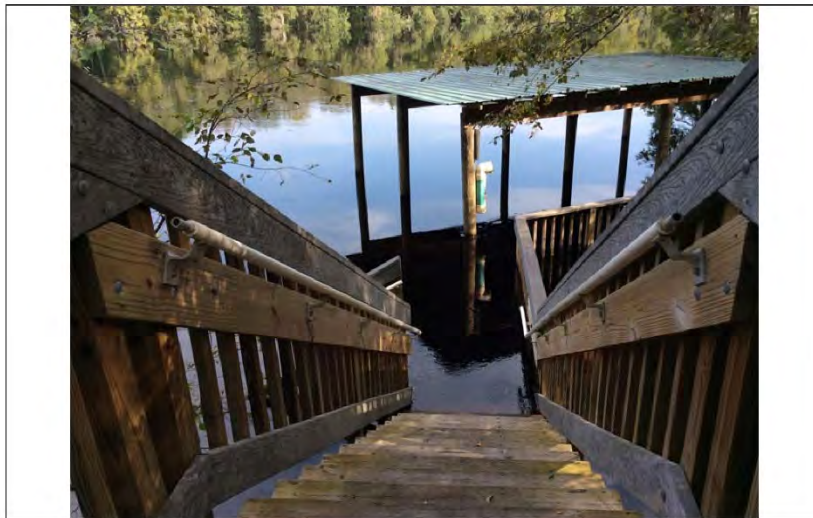
Photo No. 16. Flooding at dock location (September site visit). View to the north.
