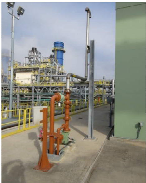
STG Seal Oil Vapor Extractor Vent
