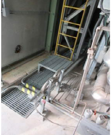
Steam Turbine HP/IP/LP Hydraulic Controls
