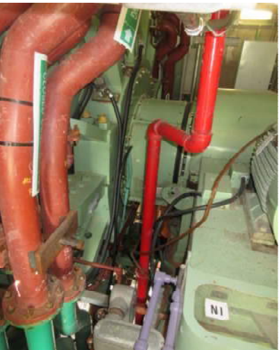
ST Generator Inboard Bearing
