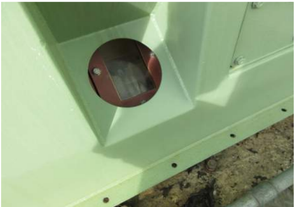
ST Generator Outboard Bearing
