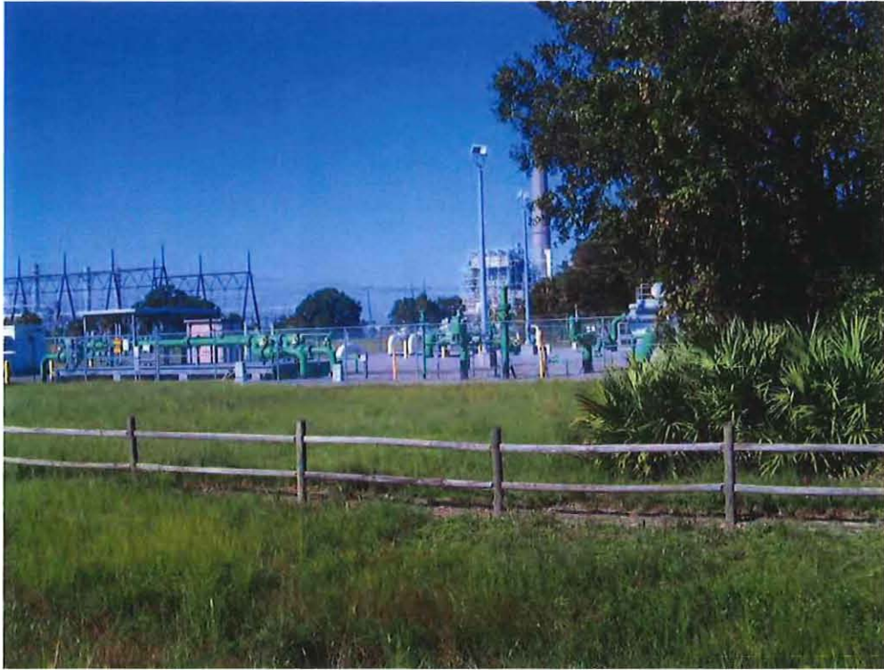
Photo 1 – Looking West at Existing Gulfstream Gas Yard
