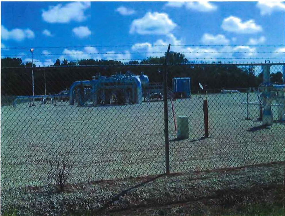
Photo 2 - Looking North at Existing FGT Gas Yard
