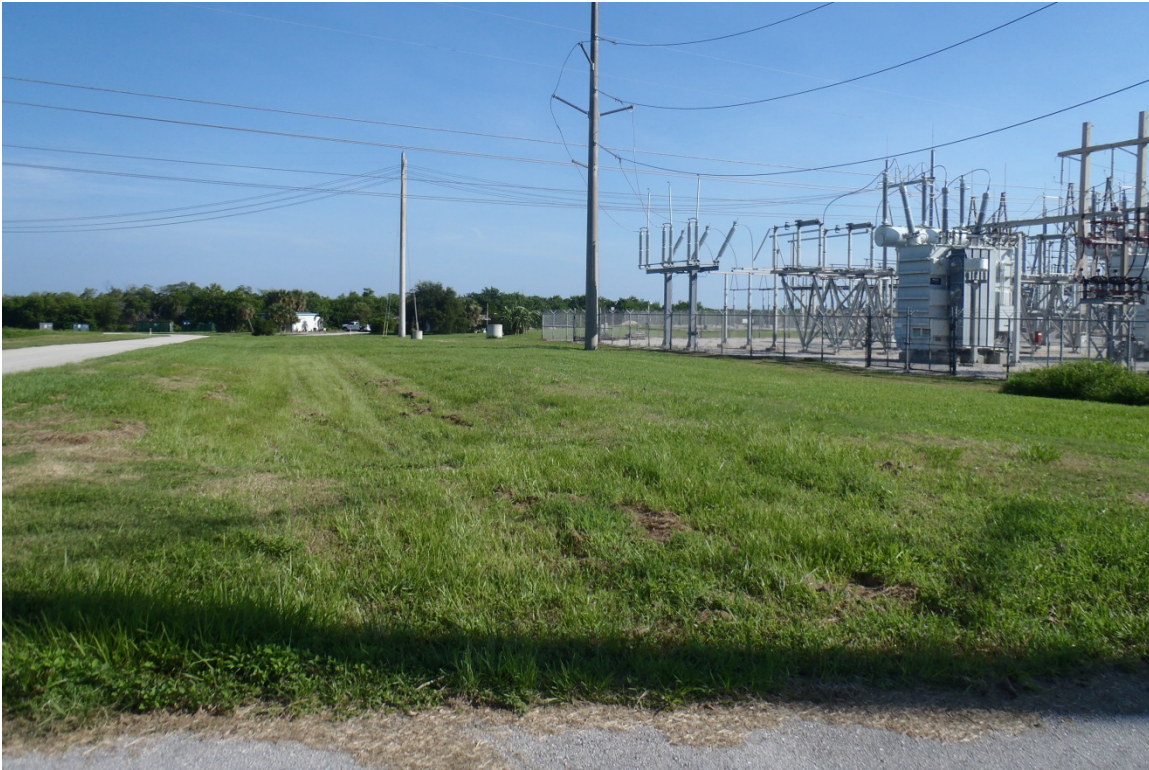
Figure 3. Existing conditions at St. Lucie Substation, facing north.
