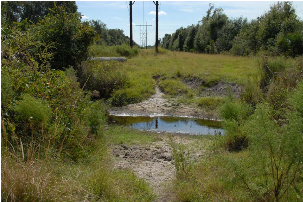
Looking south at the existing low water crossing showing eroded banks, upland plants growing to bed of drainage.
