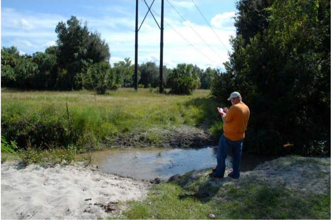
Looking north at the existing low water crossing illustrating disturbed nature of proposed crossing area, erosion, and sedimentation.
