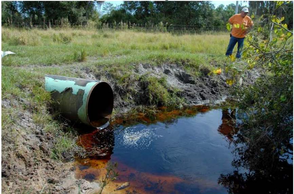
Looking Southeast at the downstream end of the existing culvert to be replaced. Note eroded banks.
