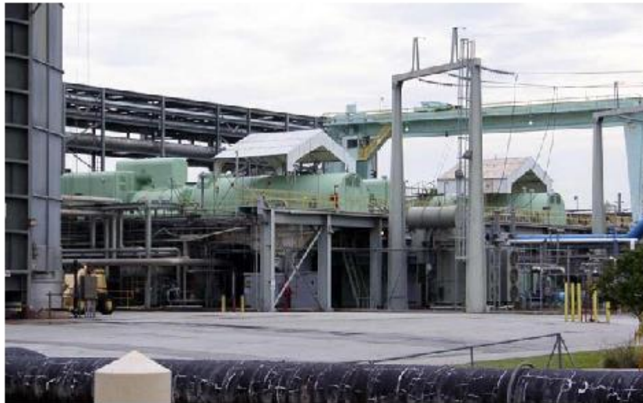
BD6978 Steam Turbine Units 4 & 5, (green painted cylindrical equipment) looking southwest (photo: FPL archives - date not recorded.)
