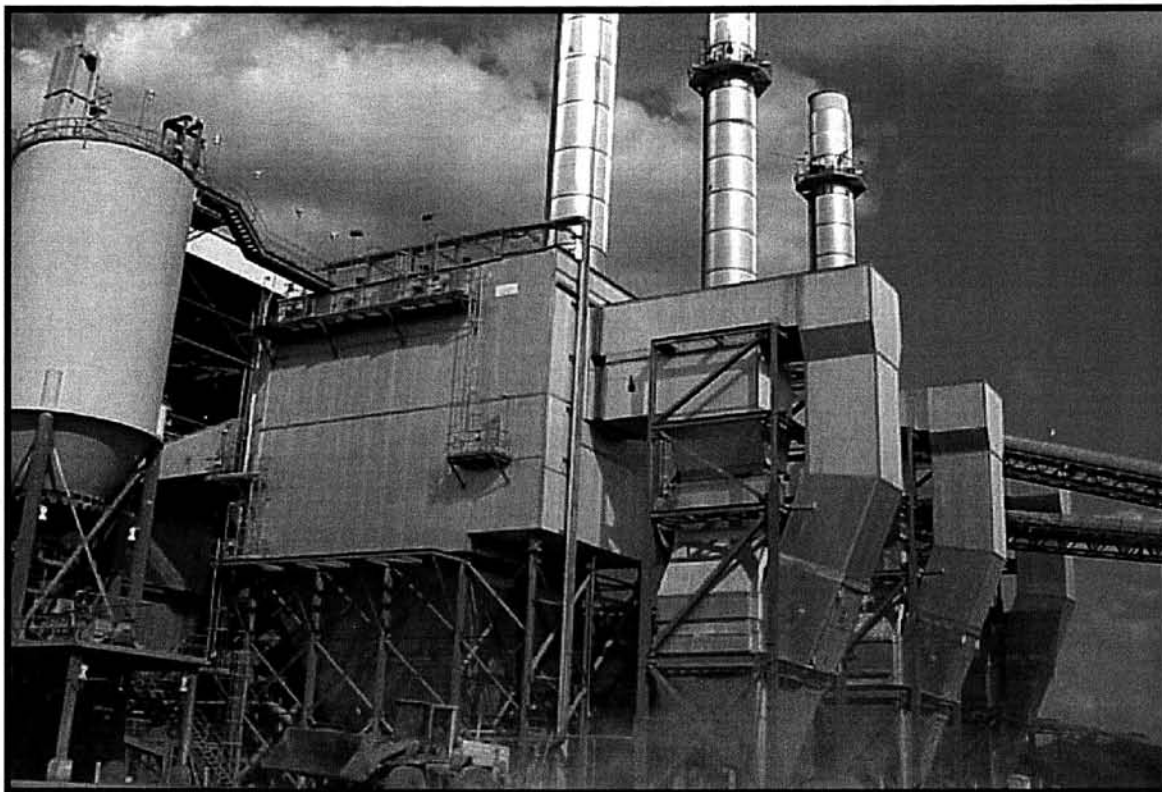
Figure 3.2-3e. NHPP Boilers Electrostatic Precipitators (ESPs).
